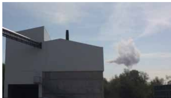
Fig. 6 – Look of the stack at normal boiler operation
